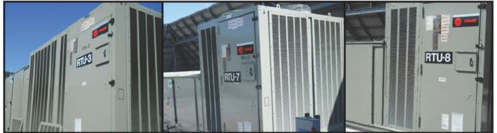
CHRISTUS St. Michael used a variety of high efficiency units to improve performance & increase energy efficiency.
